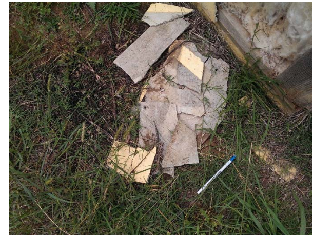
Photograph 18: Suspected ACM fragments observed near toilet
