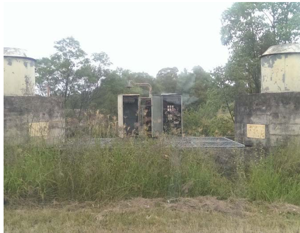
Photograph 29: Flood gate near stockpile
