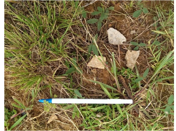
Photograph 9: Suspected ACM fragments observed next to 2 storey W02 structure
