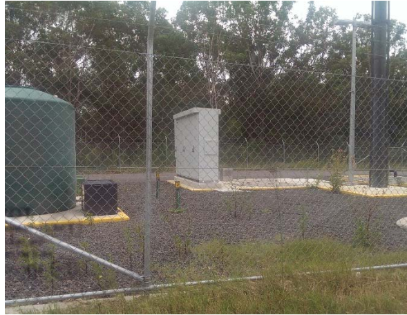
Photograph 32: Temporary sewer pump storage station on Jordon Springs connector road
