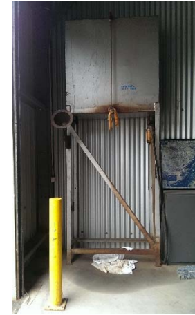
Photograph 21: 500 L diesel tank with some staining observed on the floor
